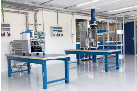
Chiller Repair Center
